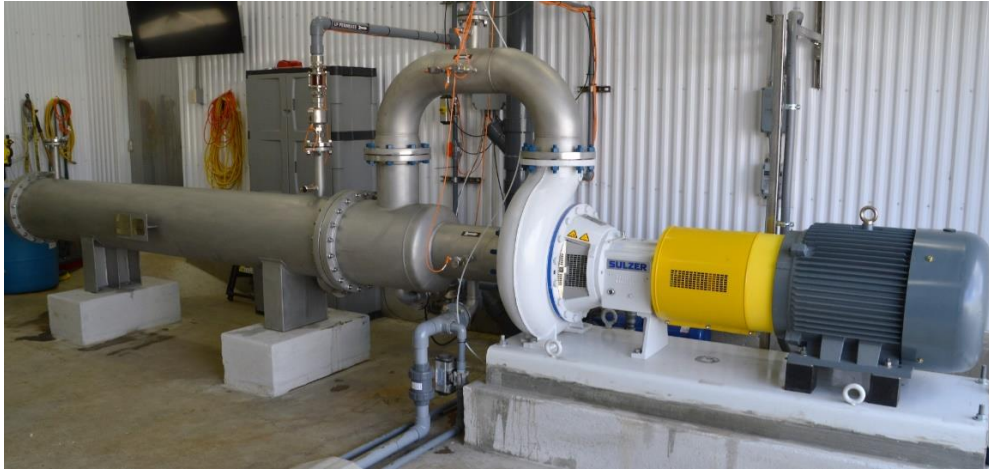
Picture of commercial ultrafiltration unit processing dairy manure in Sheboygan Falls, WI.
